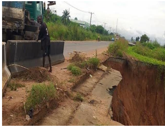
Figure 11: Erosion Spot Along Port Harcourt Road Owerri Source: Field Study, 2025
